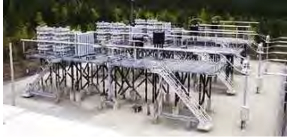
Figure 26: A three-phase series capacitor for a EHV transmission line. Warranted economically under most circumstances, installations like this pay back over many years but would be difficult to mandate only for GIC mitigation.
